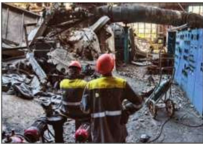
Workers standing among debris in a damaged thermal power plant in Ukraine after a Russian attack on Thursday
